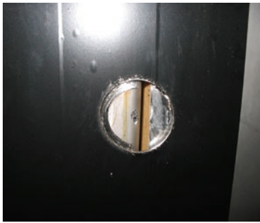
Figure 7. A hole drilled through the reflective steel revealed the insulation void.
